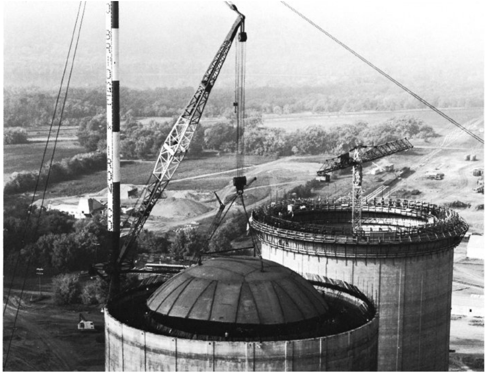
FIGURE 2.75 (Photo courtesy of CBI Industries Inc.)
