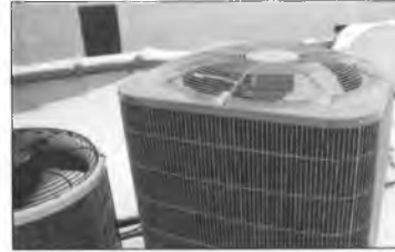
Air conditioning systems © The McGraw-Hill Companies, Inc./Jill Braaten, photographer.
