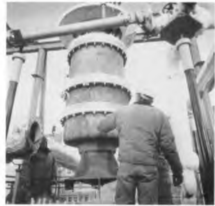
FIGURE 7–30 A 1.0-MW liquified natural gas (LNG) turbine with 95-cm turbine runner diameter being installed in a cryogenic test facility. Courtesy of Ebara International Corporation, Cryodynamics Division, Sparks, Nevada.
