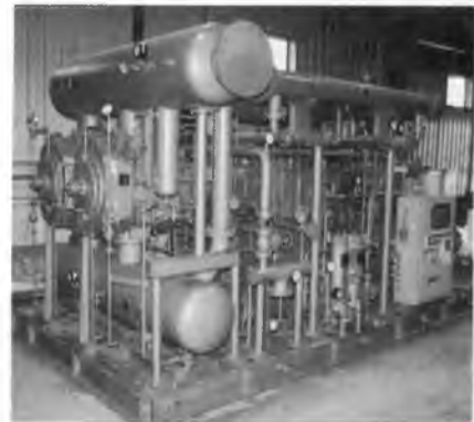
FIGURE 7–71 A 1250-hp compressor assembly. Courtesy of Dresser Rand Company, Painted Post, NY.
